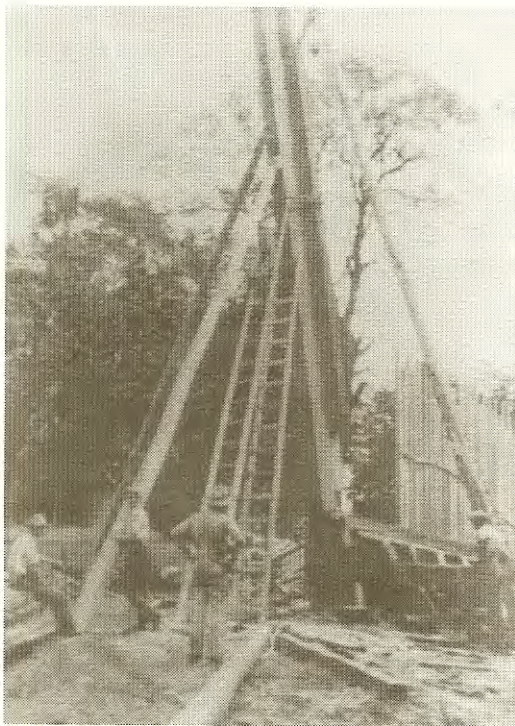
Bowsprit of a Smith & Terry barge being constructed at the Bethel Shipyard. These were ocean going barges.
