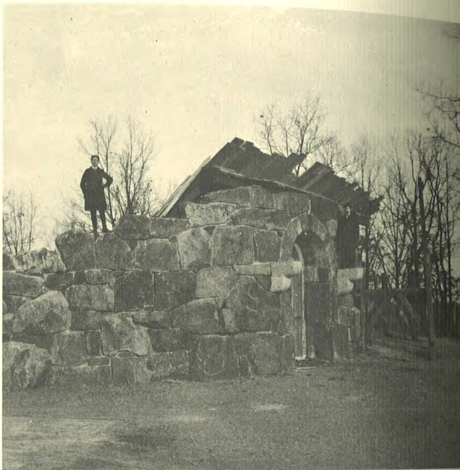
This picture of Rockford Tower under construction gives a sense of the tower's size. The door has been installed, but most of the stonework has not yet reached that height. Scaffolding is visible at the far right. (Courtesy of the Historical Society of Delaware.)
