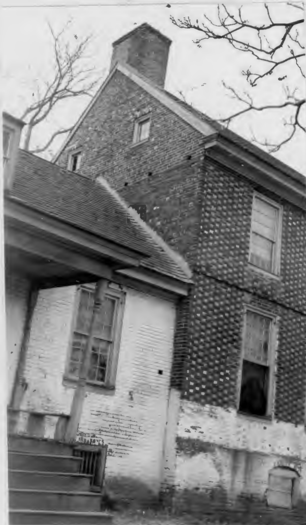
11. Detail of front and gable end at main end of building, and brick construction of front middle wing.
