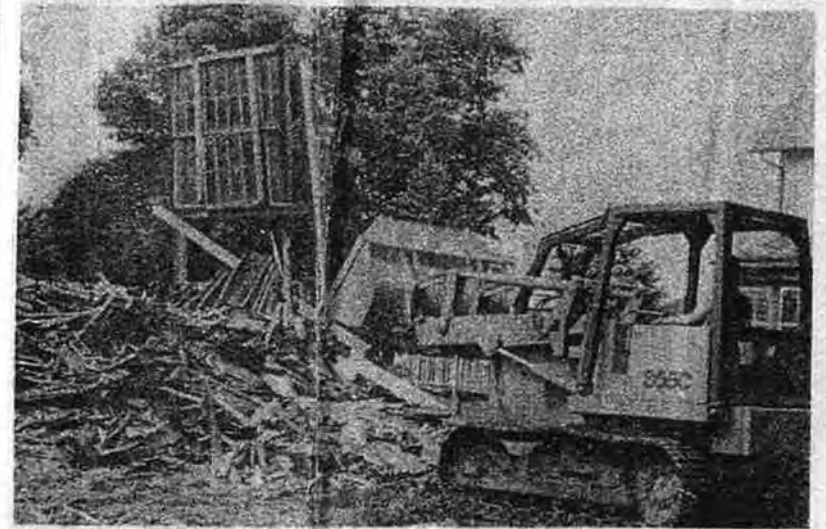
A demolition crew razed the former St. John the Evangelist Church on Valley Road in Hockessin last week.
