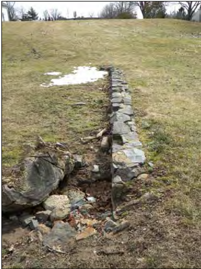
View of the remnant stone wall, looking south. Note the debris at the drainage basin.
