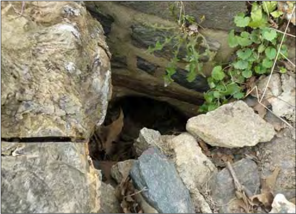
Detail of the failed 12-inch terra cotta pipe at the northern end of the stone wall. Once a part of the drainage system along Greenbank Road, this pipe outlet no longer functions.
