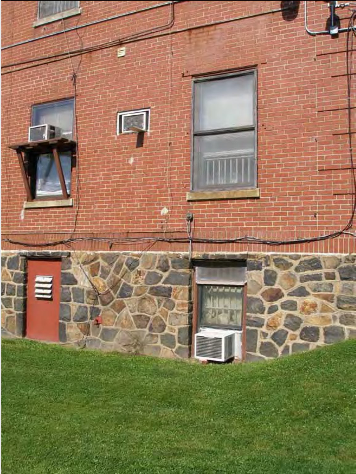
Detail of the foundation, brick cladding, and fenestration at the northern end of the east elevation.
