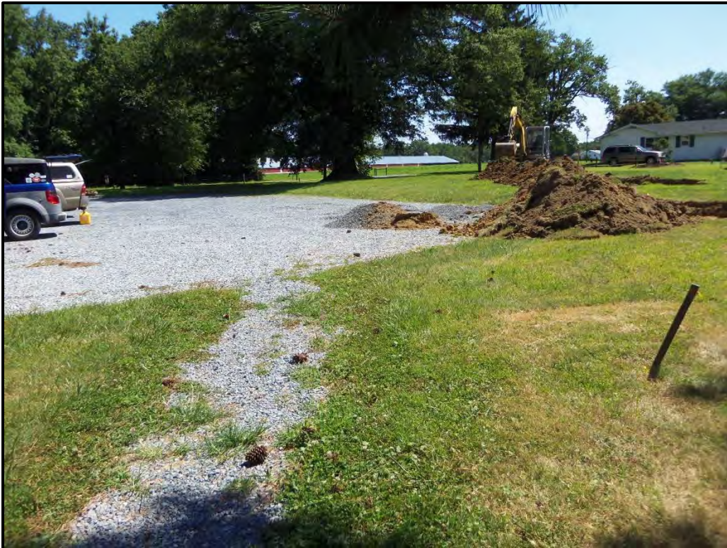
Figure 9. Trench excavation from the southeast corner of the parking lot toward the northeast
