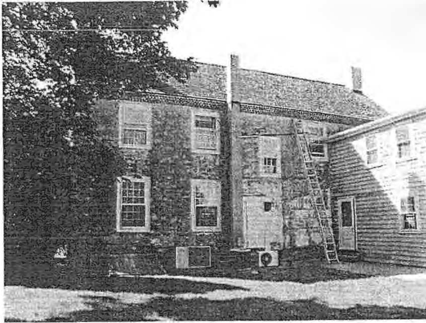
Figure 4: Perspective of the east elevation of the main block and the south elevation of the addition. The area under the ladder shows evidence of one-story shed addition with shelving affixed to the wall. (See Appendix B, photographs K-0000-5 and 6 for further documentation.)
