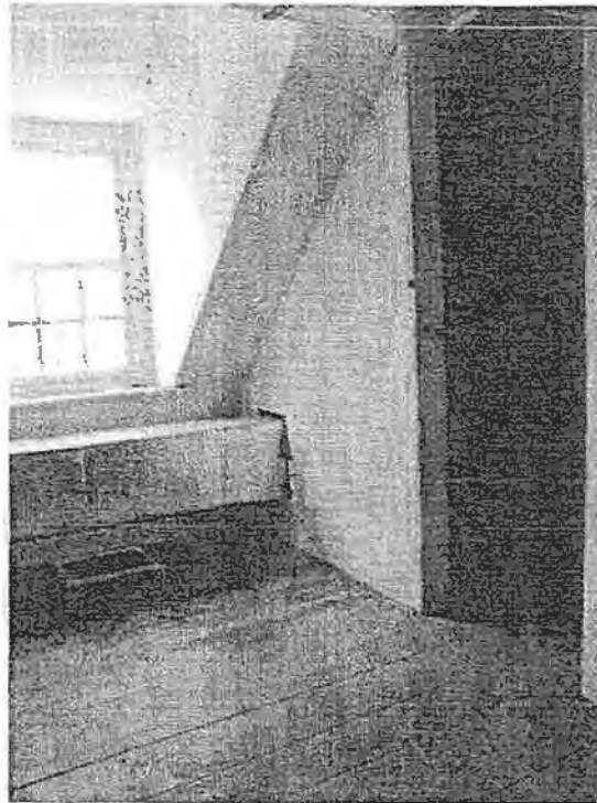
K-0000-19: Interior perspective of third floor attic landing dormer window and storage room.
