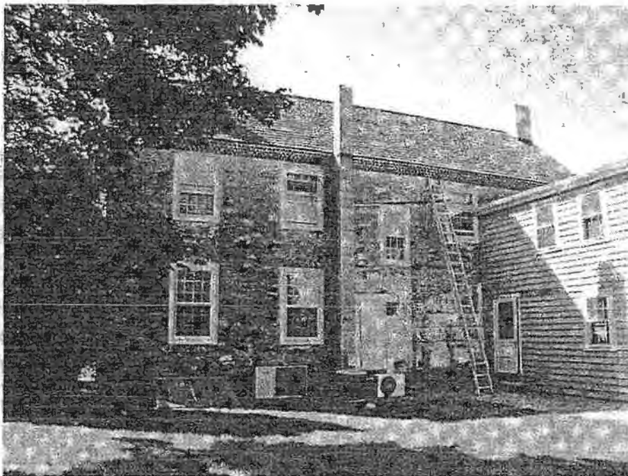
K-0000-4: Perspective of east façade looking west showing the early nineteenth century stone block, twentieth century shed addition and cement block stack and modifications to the rear entry door.
