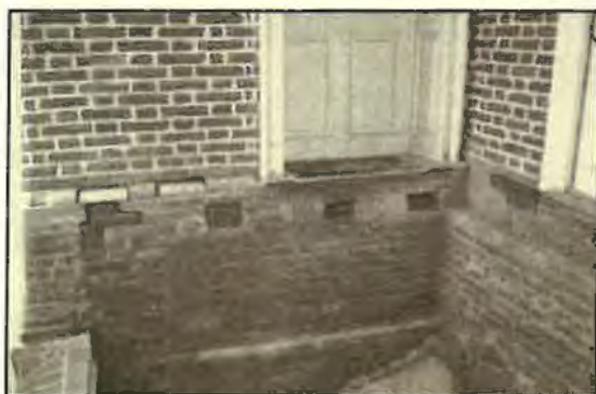
East arcade floor removed. Notice the pockets where wooden floor joists were once used.
